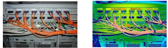
Figure 6. Visual Inspection of optical MUX-DEMUX rear cables reveals the existence of electrical anomalies (Sample 2) a) RGB regular image, b) Thermal Image
